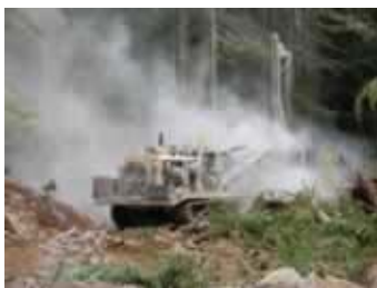
Rock drilling without dust controls.
